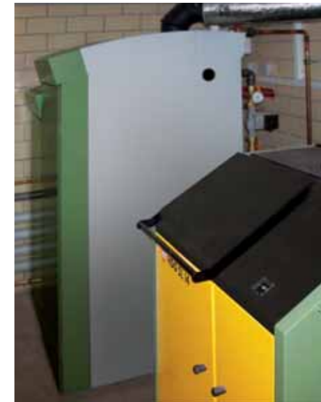
The HDG SL works very well as an auxiliary boiler. Shown here next to an HDG Pelletmaster.
